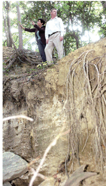
County Council members Pam Weidle, left, and Ron Dillon survey the runoff damage at Cypress Branch. By Joshua McKerrow -- The Capital
